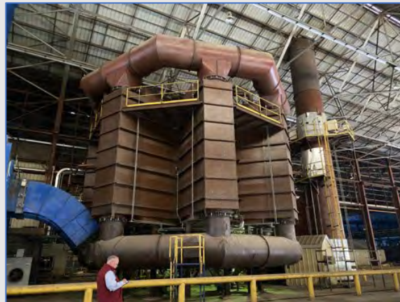
Main Plant Interior
